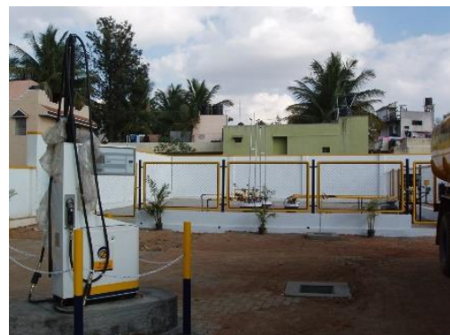
Underground LPG storage tanks at an Autogas station
