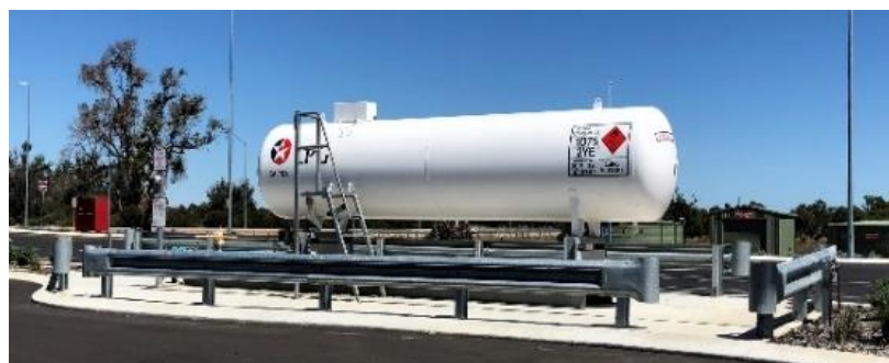
A 7.5kl above ground LPG tank servicing an Autogas site
