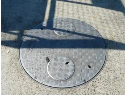
Underground Autogas tanks look no different to diesel and gasoline ones Source – D J Batchen, Australia
